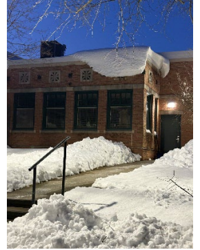
“Eyelash” hanging off the roof
