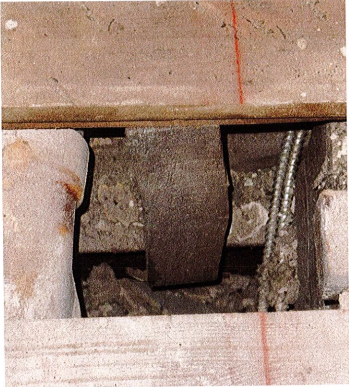
Photo 5: Existing observed buckled joist
