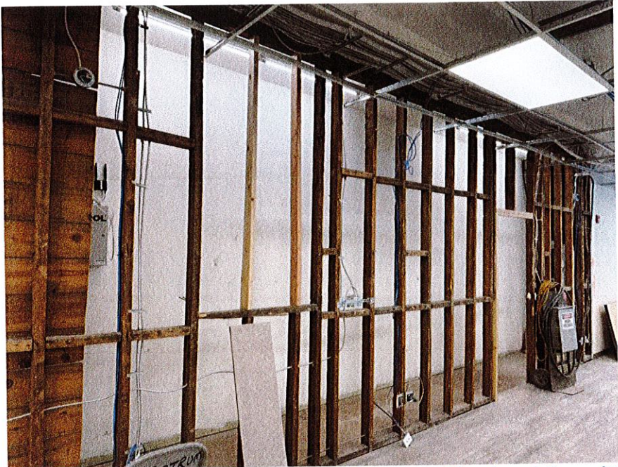
Photo 1: Existing wall planned for removal, found to be a bearing wall based on existing conditions
