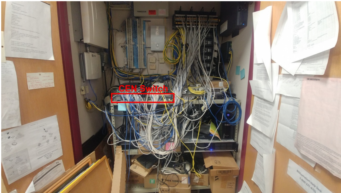
North Branch Library CEN Switch
